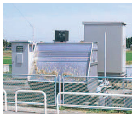
Site: Pumping station (Iutake river water)
