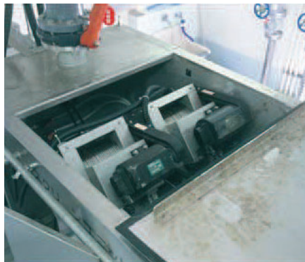
Site: Agricultural community waste water treatment plant
